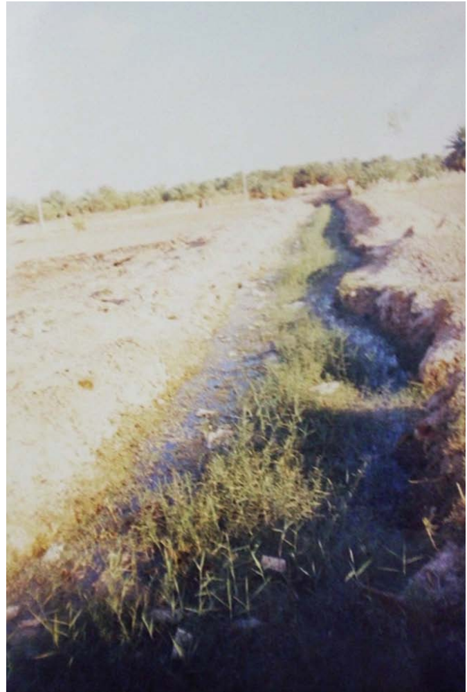
Photo 3: Erosion of drain.
